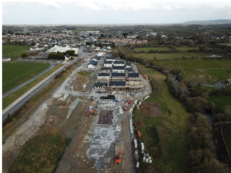
Site progression – View from south of site (Foundations for Phase 3 under construction)
